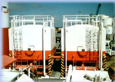
Drilling Mud Mixing Tanks
