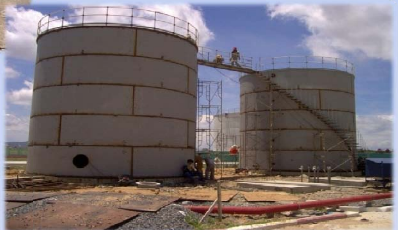
Water Storage Tank, Vietnam
